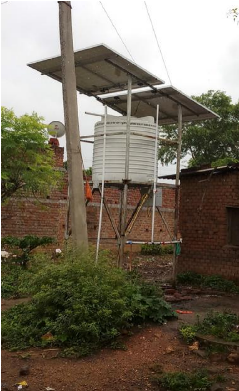
Photo: Solar Water Pump and Water Tank, GP Soso (Ramgarh, Jharkhand)
